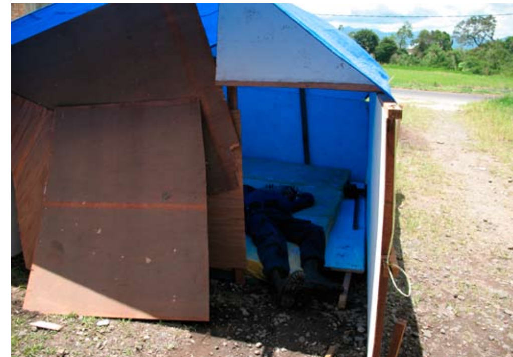
Figure 20. A damaged local fire station building, with the cracked URM wall is shown in the top photograph, and temporary shelter for five firefighters is shown in the bottom photograph.
