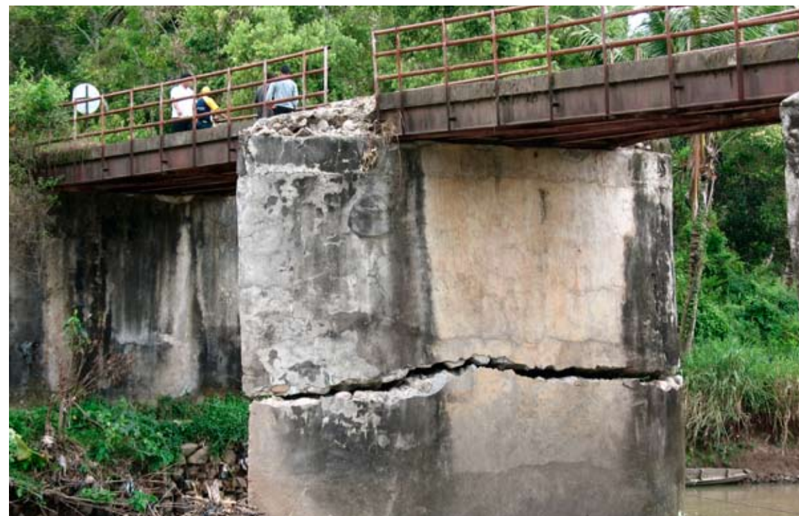
Figure 16. The photographs show failure of piers for the concrete bridge. A heavy deck and bents contribute to high seismically induced force experienced by the bridge, which caused the brittle shear failure in one bent and rocking at another. This bridge is near collapse, and traffic has been redirected.
