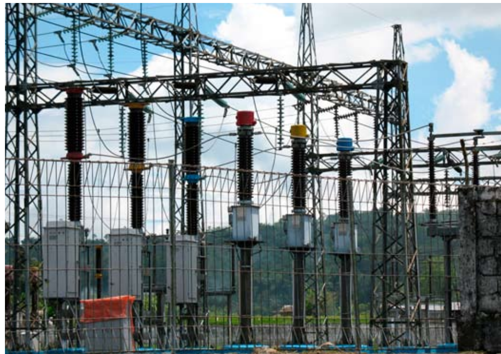
Figure 19. The local electric substation and its bushings are shown above. One bushing fell and caused a blackout for a few days.
