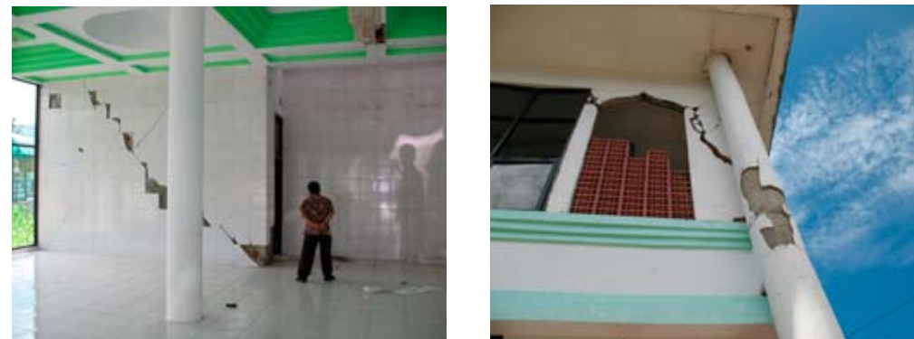
Figure 11. These photographs show spalling of concrete from tall, slender column at the story level and shear failure of the interior URM wall. Note that walls are placed on the back side only, and thus the building is torsionally irregular.
