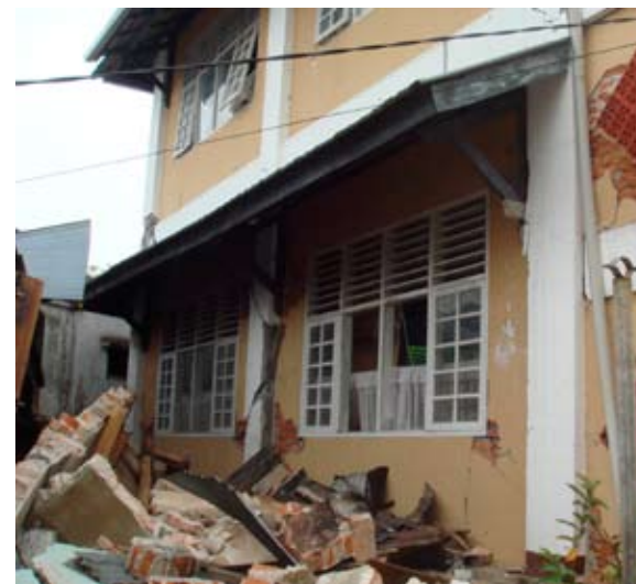
Figure 7. The presence of URM infill dramatically alters the seismic response of concrete frames. The infills reduce the clear height of the columns from story height to the height between solid infills. This short-column effect prevents development of full flexural capacity and induces brittle shear failure.
