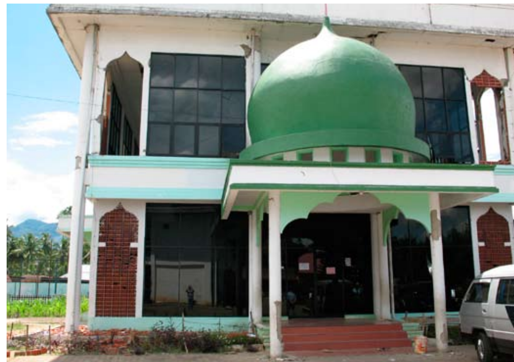
Figure 10. This photograph shows typical mosque construction. Note the slender exterior concrete columns. This building was constructed in the mid-1990s.
