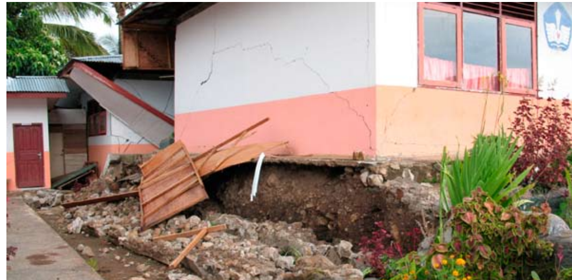
Figure 13. The photograph shows unreinforced retaining wall failure of a school building. Note the diagonal shear cracks on the URM walls at the side of the building.
