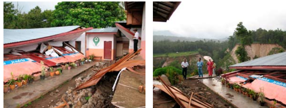
Figure 14. These photographs show out-of-plane collapse of URM walls. The walls were not adequately anchored to the foundation or roof diaphragm to restrain the URM walls. The Sumatra Fault is shown in the near distance. The roof diaphragm, perimeter concrete beam, and columns were weak.
