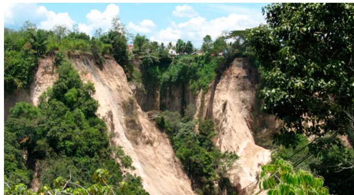
Figure 23. As shown in these photographs, the earthquake also caused noticeable ground rupture both horizontally and vertically. Note the large section of slope instability next to the Great Sumatra Fault in the bottom photograph.
