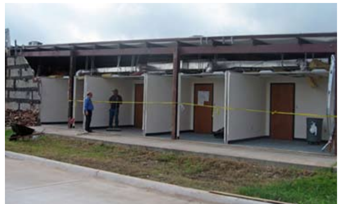
FIGURE 5. Roof damage was common throughout the area and some properties, such as this structure, lost entire walls as well.
